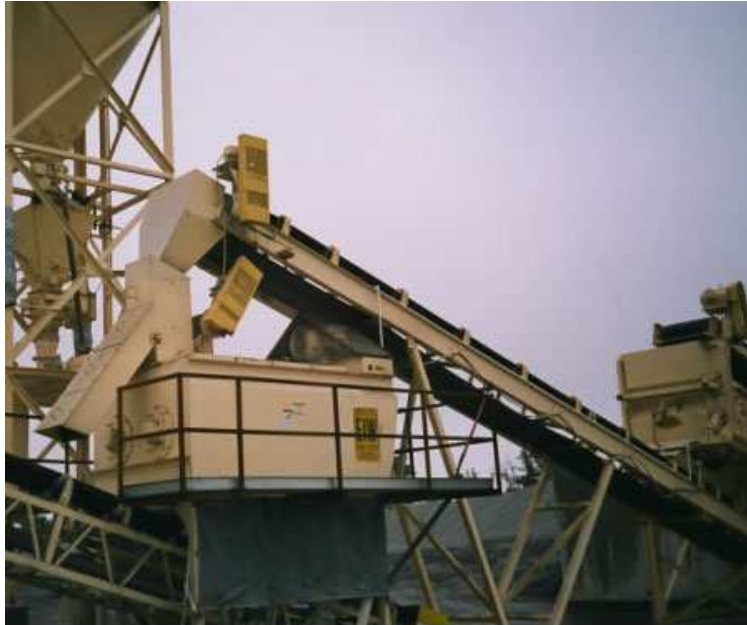
Figure 29: Pugmill used to mix hydrated lime with the wet aggregate in South Carolina (from [145]).
