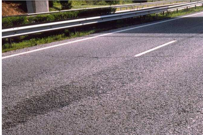
Figure 7: Aggregate stripping as a consequence of moisture induced-damage (from [45]).
