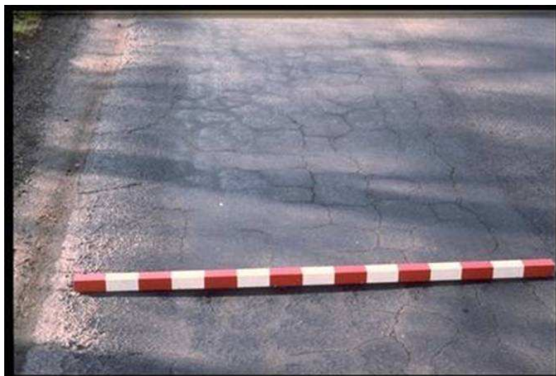
Figure 18: Fatigue cracking (= alligator cracking) in an asphalt mixture (from [45]).
