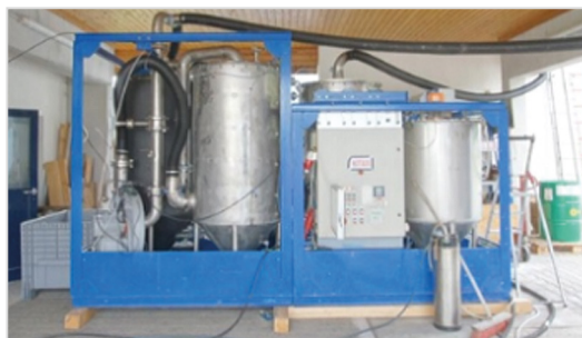
CO 2 scrubber used at the waste water facility at Bad Orb, Germany.
