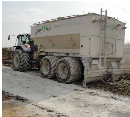
Figure 4.13 – Mounted spreader (© Lhoist)
