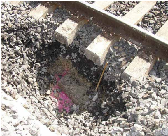
Figure 7.3 – Test pit showing contaminated ballast and a reinforced concrete slab at the bottom of the pit (Herle, 2005)
