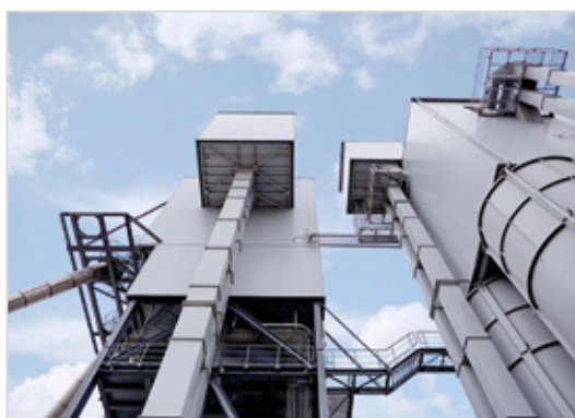
Supply and return bucket elevator for the lime circuit and RDF delivery.
