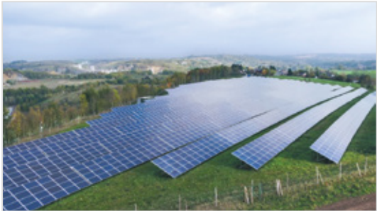
Solar panel farm at Moha (Wallonia).
