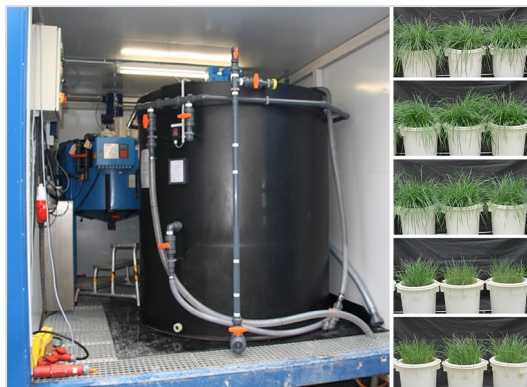
Pilot plant for the recovery of Phosphate from sewage sludge and planting tests performed by University of Bonn (DE).
