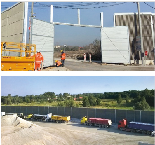
Noise barrier at Miedzianka (Poland).
