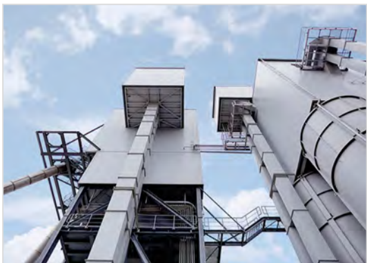
Supply and return bucket elevator for the lime circuit and RDF delivery.
